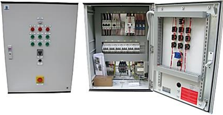
Figure 7.1 – Thyristor Control Panels
