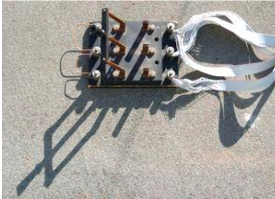
Figure 2.1 - Triple Pole Single Throw (TPST or 3PST) knife switch used to short the windings of a 3 phase wind turbine for braking purposes. Here the switch is shown in the open position
